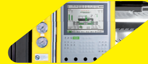
Automatic control Austria made KEBA controller model 2880
